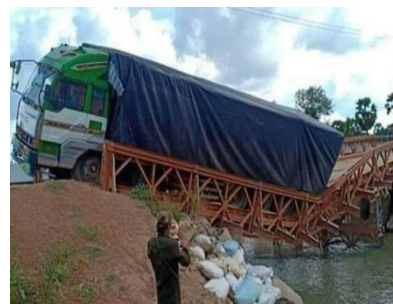
Overloaded truck damages bridge
